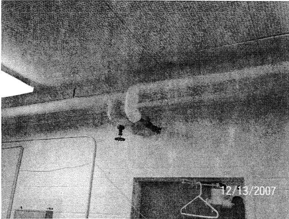
Photo 1: Pipe and fitting insulation in Maintenance Office
